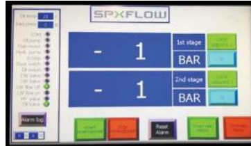
PLC Control Panel for Homogenizers
